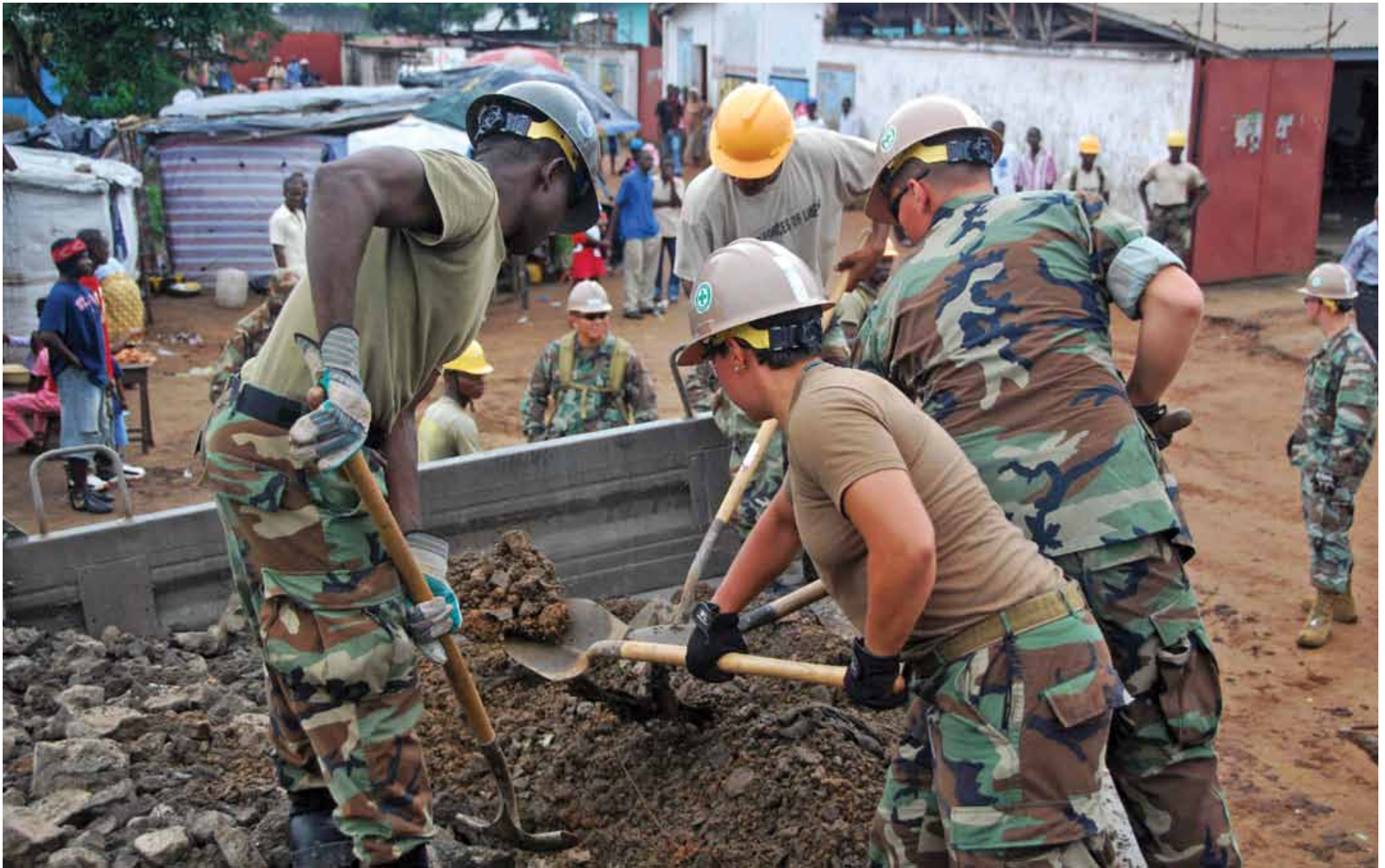
PEDIATRIC WARD - Armed Forces of Liberia (AFL) and U.S. Navy Seabees from Naval Mobile Construction Battalion (NMCB) 3 load dirt and debris into an AFL truck for removal from a building site at Redemption Hospital in Monrovia, Liberia, in September 2009. The personnel were building a pediatric ward and laundry facility as part of Africa Partnership Station. (U.S. Navy photo by Petty Officer 1st Class Dan Meaney)
