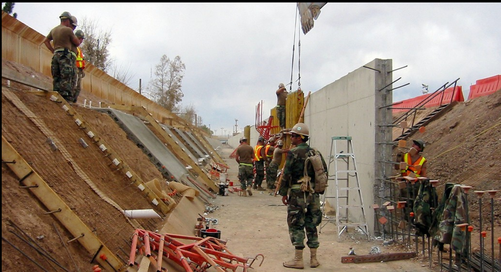
Arizona (March 14, 2009) Seabees assigned to Naval Mobile Construction Battalions construct a 1,500 foot-long concrete-lined drainage ditch and a 10 foot-high wall to increase security along the U.S. and Mexico border in Douglas, Ariz. (U.S. Navy photo by Steelworker 1st Class Matthew Tyson/Released)
